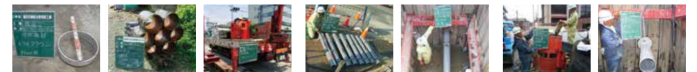
Metal crown Steel pipe Hydraulic power unit Insertion of main pipe Injection of filling material
